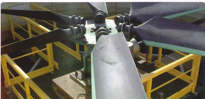
Entrance platforms Cooling tower
