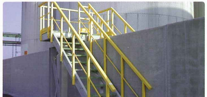
Step over platform Chemical tank storage
