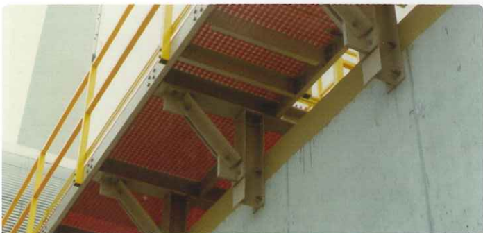
Platform Power plant
